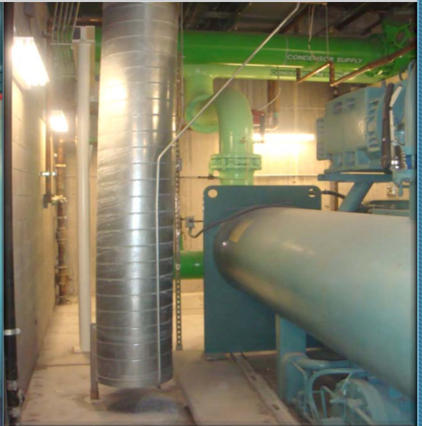
Existing Un-Supported Installation
